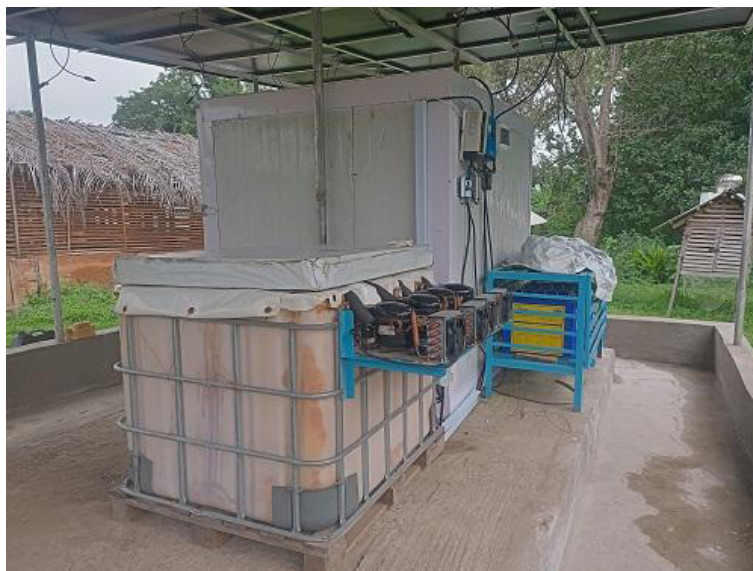
Figure 3: The Back view of the solar cold room showing the cooling unit and battery system
