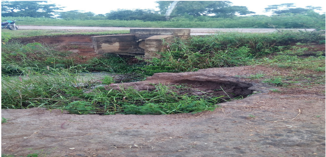
Plate 5: A typical example of gully hazard where a bridge is about to collapse at Mugau 2
