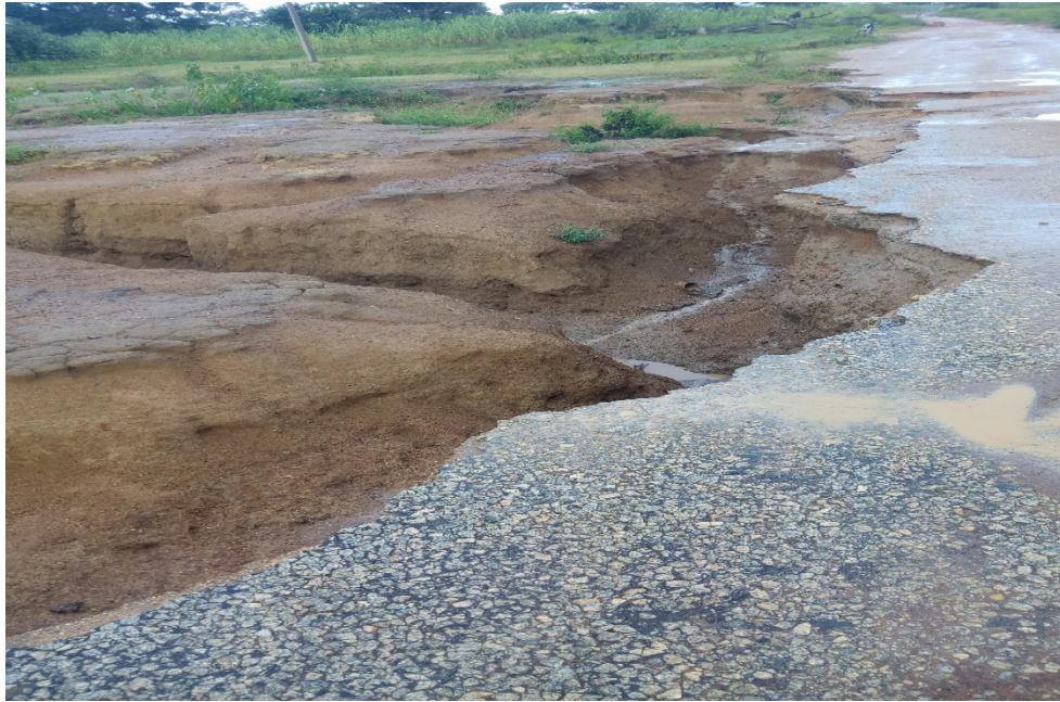
Plate 2: Road nearly cut off by a gully erosion at Mugau 2
